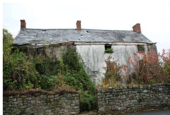
Fig.35 Caerwent House: a significant building in the Conservation Area is in a very poor condition
