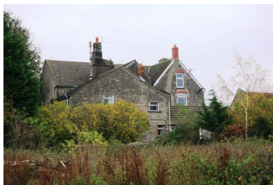
Fig.20 The prominent roof slopes of Great House farmhouse with modern concrete interlocking tiles
